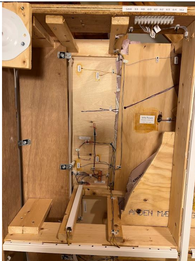
Kabling under stationen
